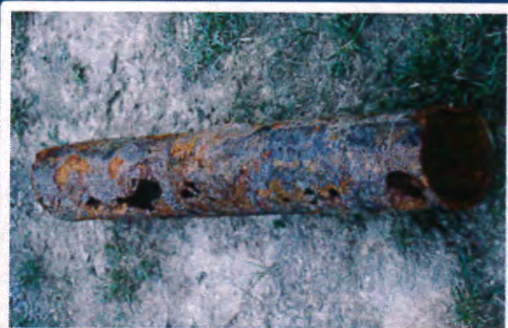
Water pipe from Letcher County, Kentucky, coal camp, installed early 1900s.
